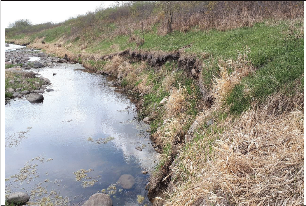
Photo 3. Eroded bank downstream of Station 1.
